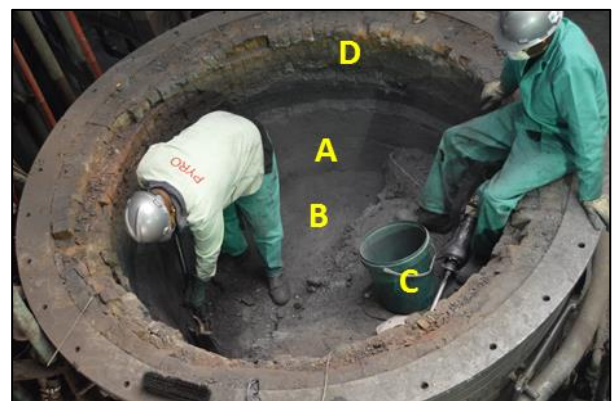
Fig 9: Removal of the burden. A-carbon-based sidewall refractory, B-carbon-based hearth lining, C-bucket for removal of material, D-magnesia bricks
