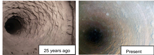
Fig. 1: Appearance of inside of past (25 years ago) and present cement kilns immediately after shutdown.
