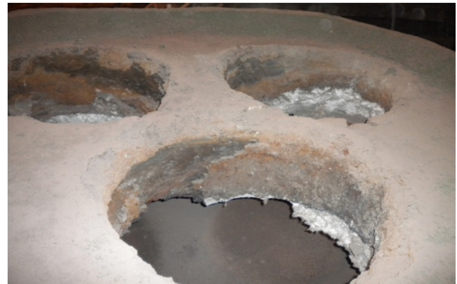
Fig. 6: Mullite bonded castable with fireclay; EAF-Delta with reduced costs and at least same performance.
