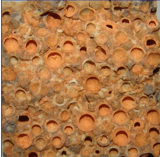
Fig. 7: Section of the LW castable using mullite based hollow balls as aggregate
