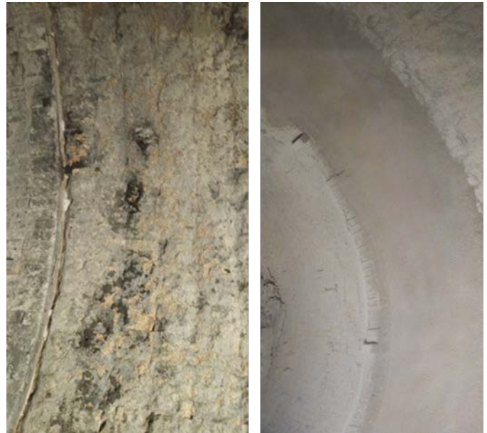
Fig. 7: Pictures of the bricks lining before castable application and the final appearance of the coated area, CEMEX Castillejo, Spain.
