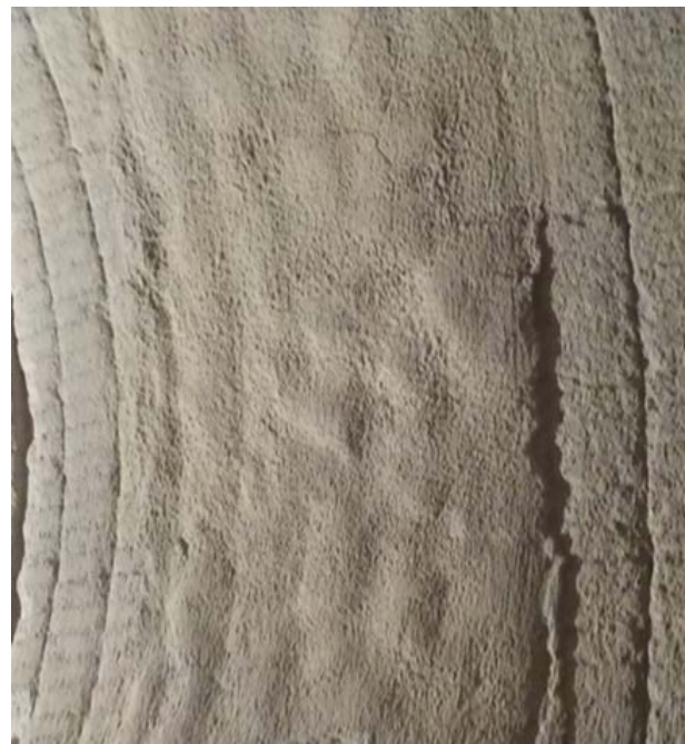
Fig. 8: Magnesia-Spinel castable coating after 5 days of operation. CEMEX Castillejo, Spain.
